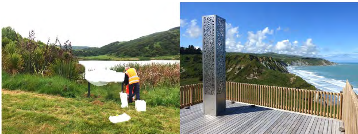
Figure 7. Installing the interpretation panel at Kate Pond and the Pou Ika at the coastal lookout platform looking northeast up the coastline.
