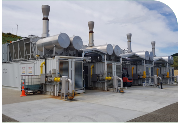
These generators convert the gas to electricity
