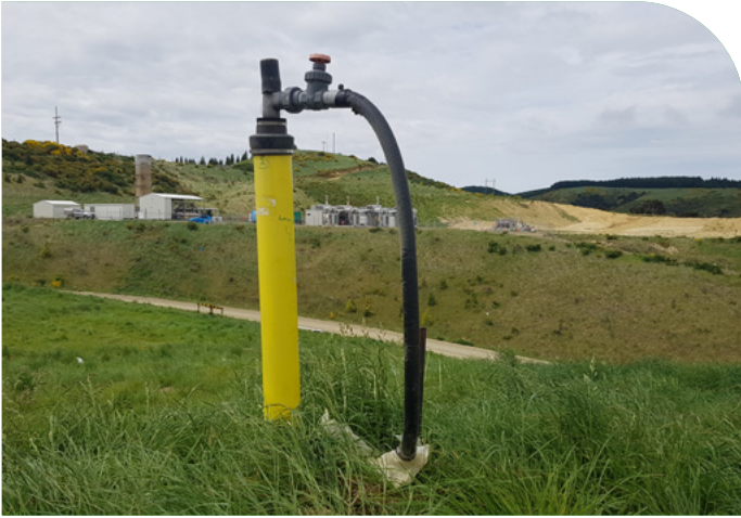
A gas well collects gas from deep inside the landfill
